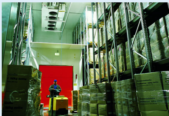
Maximum operative security with the Güntner NH 3 evaporators S-ADHN 066D/412 in a deep-freeze storage room
